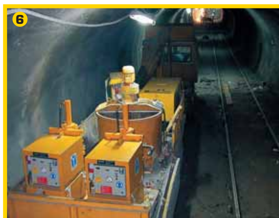
5) Grout plant with automated weigh-batching and four grout pumps for general grouting work. Bratislava.
